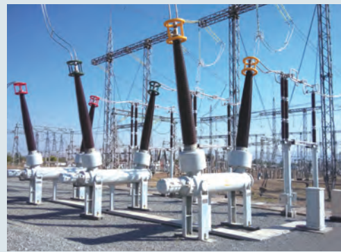
550 kV Circuit Breaker
